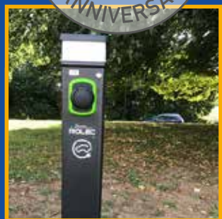
Electric Vehicle Charging Points
